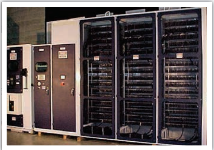
1250Hp slurry pump SRC with variable speed.
